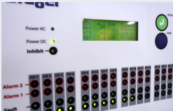
SAFETY CONTROL SYSTEMS PLC
